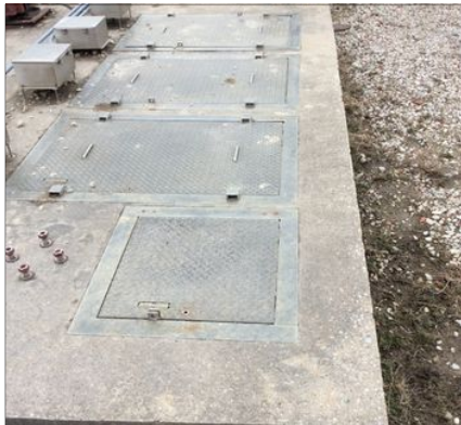
Plainview Lift Station
